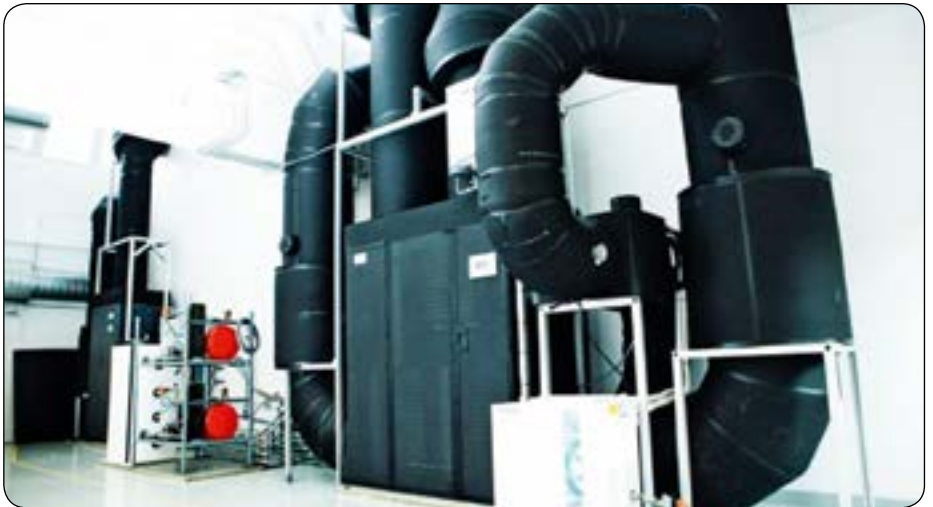
Teknologisk Instituts laboratorium for store varmepumper.
